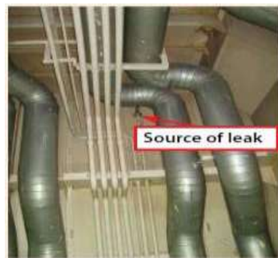
Flange joint on vent / overflow line with loose nuts located high above after exhaust manifold of main engine
