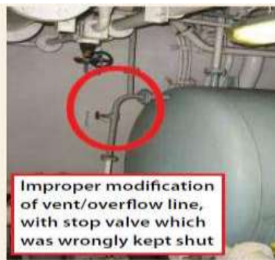
View of hydraulic header / service tank before corrective action
