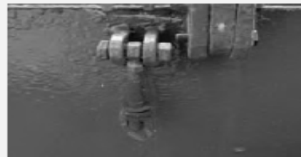
Non-standard bolt was used in place of a safer 'drop-nose' pin
