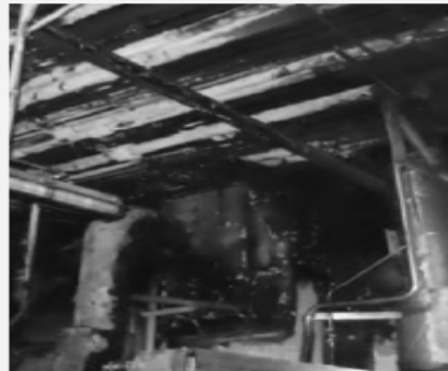
View of fire damage
