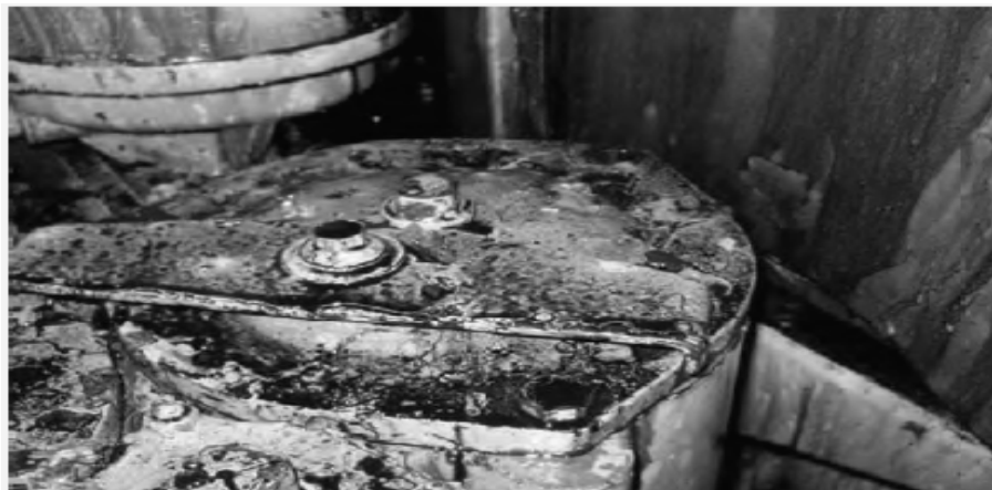
View of displaced fuel filter cover
