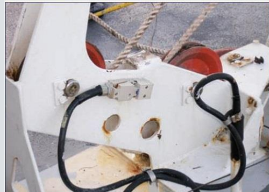
▲ Figure 1: View of proximity sensor/limit switch arrangement on davit (Note cable entry gland position raised above horizontal, potentially permitting ingress of water)
